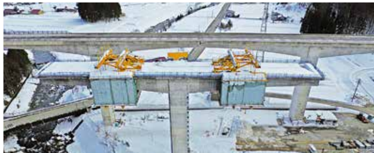
Figure-2 Arrangement of the movable hanging scaffolding system during the winter temporarily suspended period
